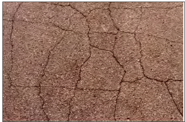
Condition 5 – Very Poor
